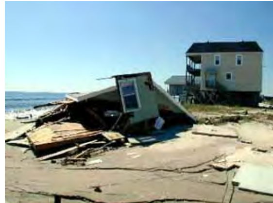
Photo 4.3 Hurricane Floyd Storm Surge Damage
