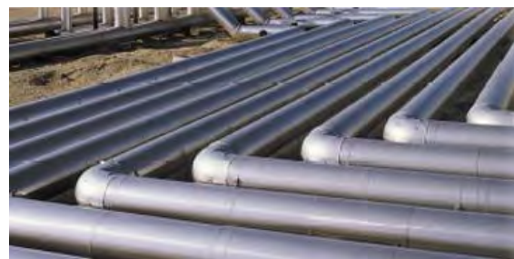
Photo 4.15 Natural Gas Pipelines
